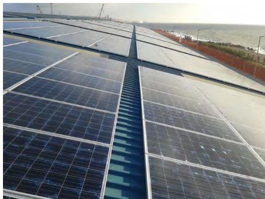
Solar panels on warehouse roofs
